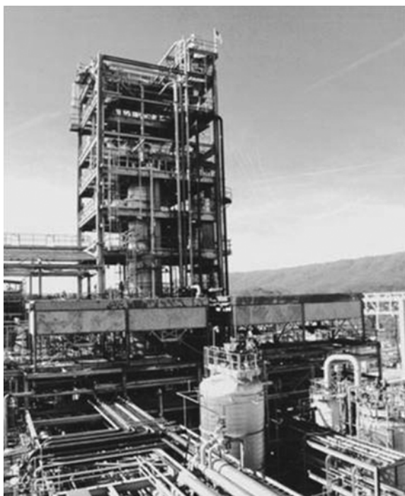
Figure 1.15. Air Products's LPMEOH process demonstration unit for methanol synthesis using syngas from coal gasification with slurry bubble column reactor, located at the Eastman Chemical site in Kingsport, Tennessee. U.S. DOE Topical Report No. 11, April 1999, under DOE contract #DE-FC22-92PC90543. Photo: courtesy of Debbie Bauer, Corporate Communications of Air Products.
