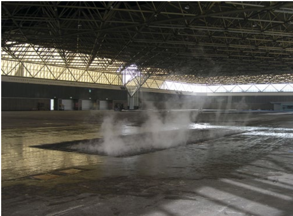
Entfernen des Asphalts, Amsterdam RAI Messezentrum I Removing the Asphalt, Amsterdam RAI Exhibition Centre, Amsterdam, 2004.
